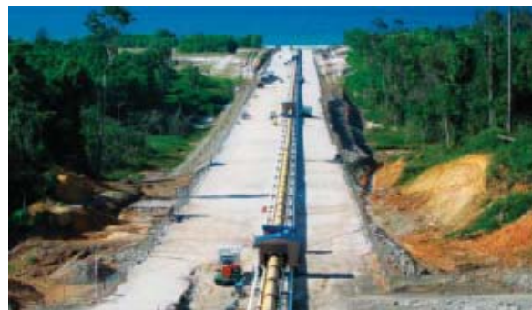
Construction of the FTL underway in a purpose-developed site near Bintulu, Sarawak
