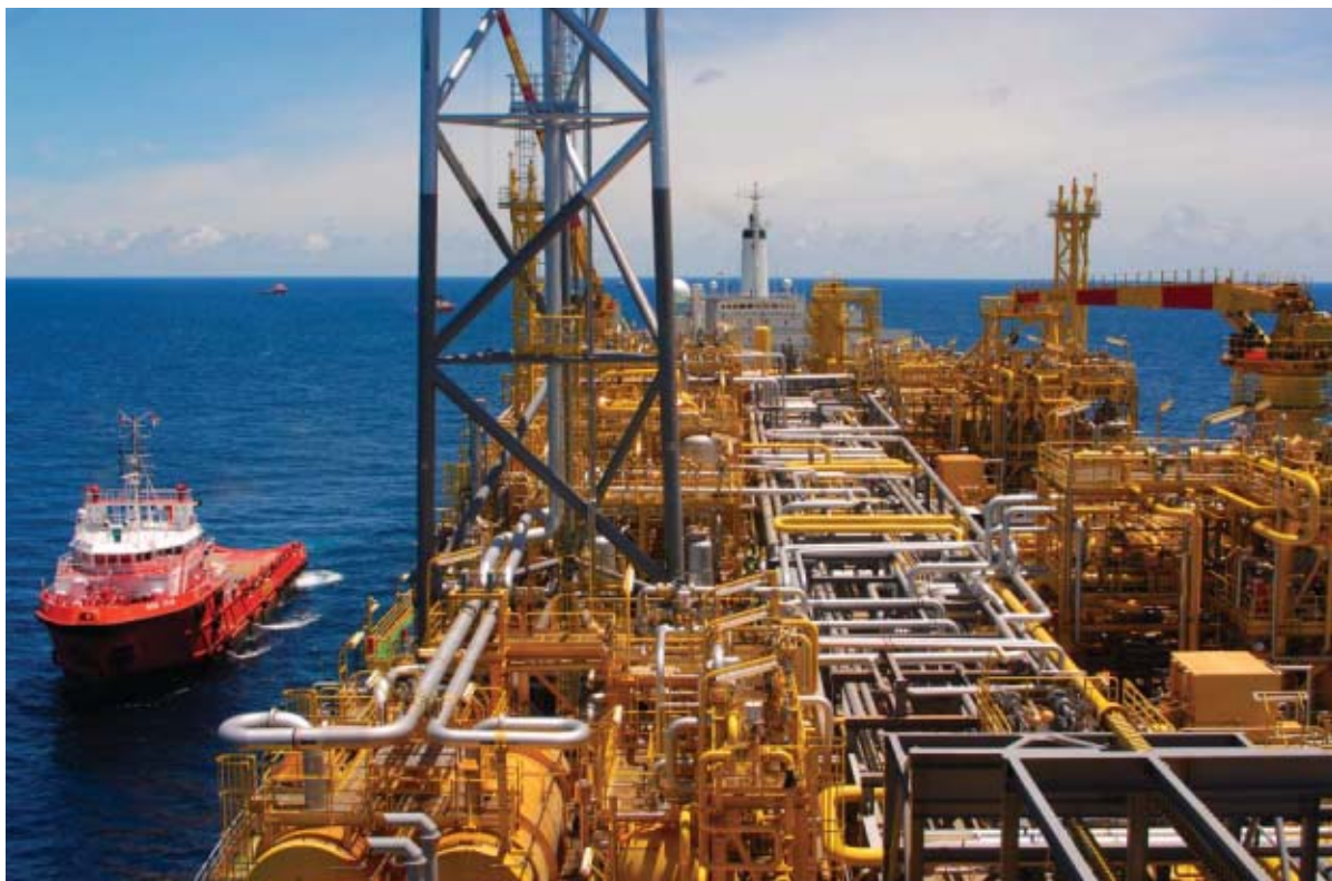
FPSO Kikeh top deck
