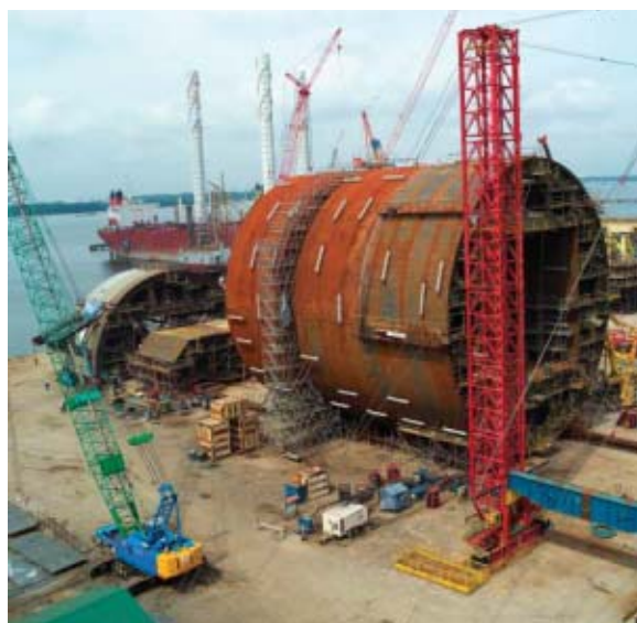
More than 100,000 management and engineering manhours were spent on Interface Management, says Oran
