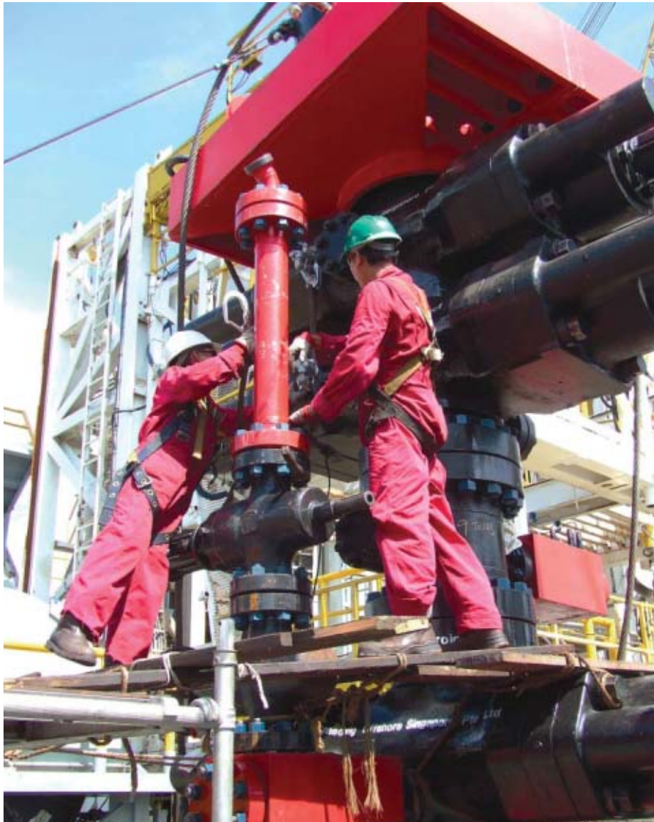
The West Setia's 16-3/4" surface blow-out prevention stack being rigged up prior to DTU drilling operations.
